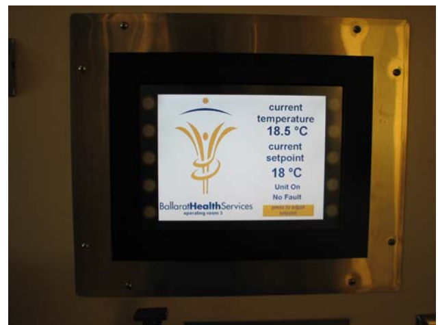
OptoTerminals provide an easy to-use-interface to the Opto 22 control system.
